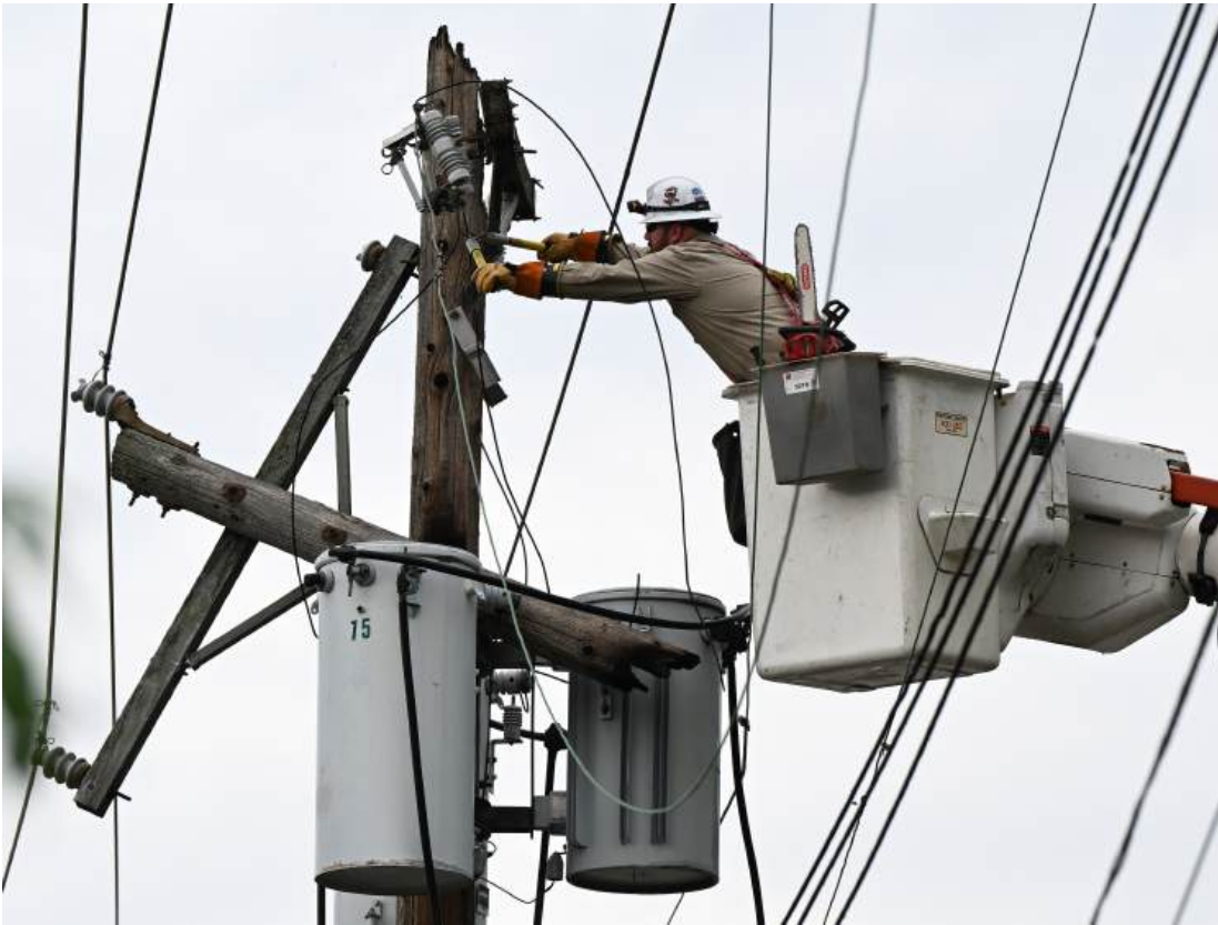
A Duquesne Light worker responds to a downed power line on the North Side on Thursday, May 1, 2025.
